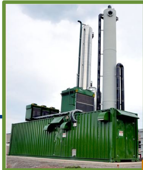
Water Scrubbing Technology
