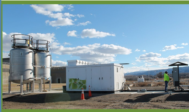
Persigo WWTP Grand Junction, CO
